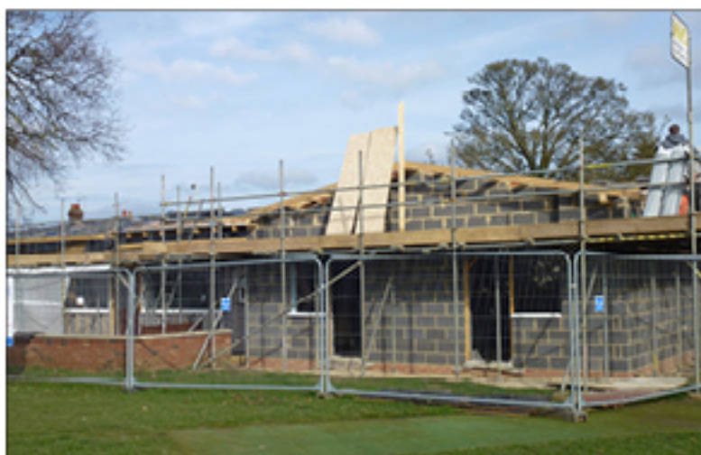
Front elevation of the club with the new changing rooms taking shape
